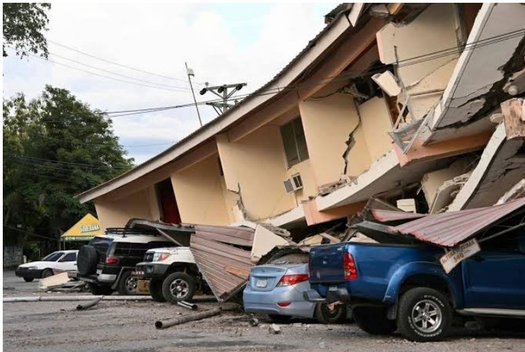
因強地動導致的建物結構損壞。(圖片來源: CBS News / 路透社, https://www.cbsnews.com/losangeles/news/los-angeles-county-search-and-rescue-deployed-to-panama-after-powerful-earthquakes/ )
